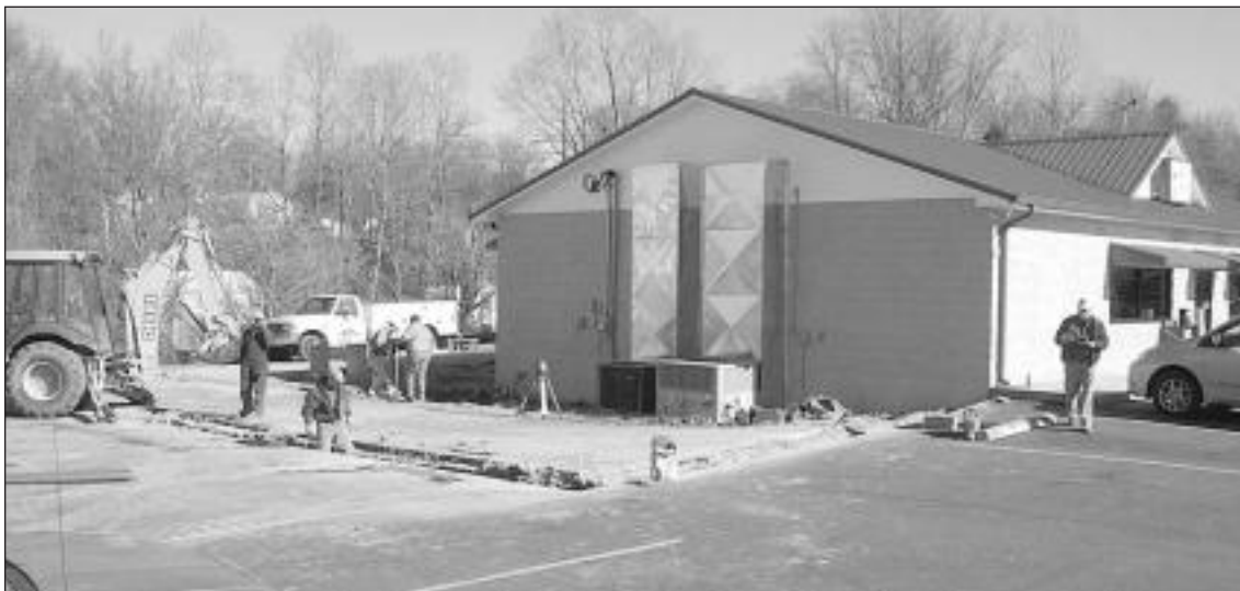
Work was being done Friday to pour the footer for the expansion of Billy's Restaurant in
